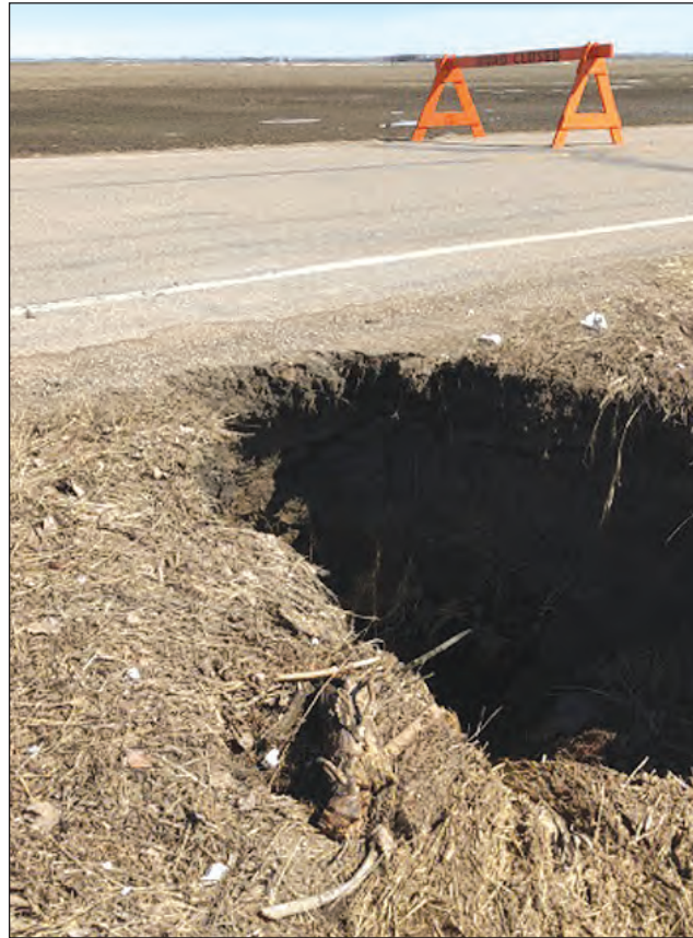
Township 14-2 , Range Road 16-0 and 15-5 – Culvert washout and repair
