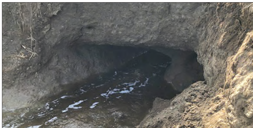
Township Road 15-0, Range Road 17-0 – Washout under Road
