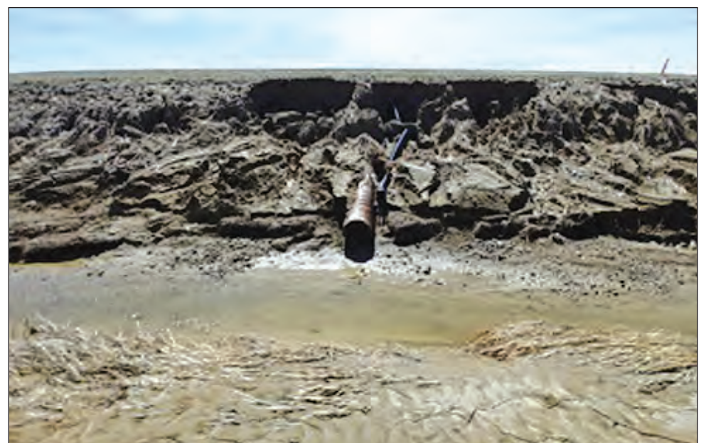
Figure 1.2: Drain Inlet Culvert on South Bank of Lateral G Big Bend Washed Out by Overland Flooding
