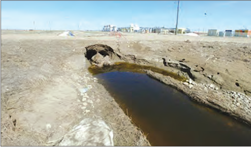
Figure 2.1: Piping Failure and Bank Sloughing at Lateral G-7 Big Bend Culvert Crossing (from South)
