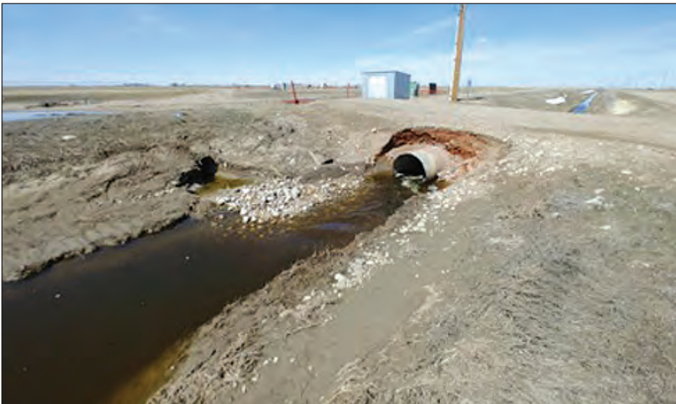
Figure 2.3: Erosion and Sloughing Around Culvert Inlet on Lateral G-7 Big Bend (from South)
