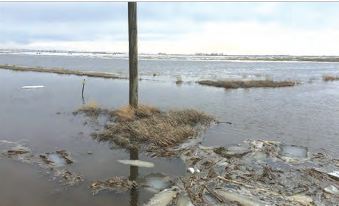
Township Road 15-0, Range Road 17-0 – Washout under Road
