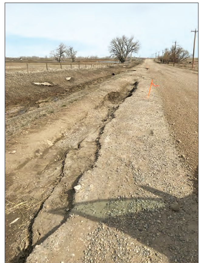
Range Road 17-2 North of Township Road 10-0 – Road Erosion (after)
