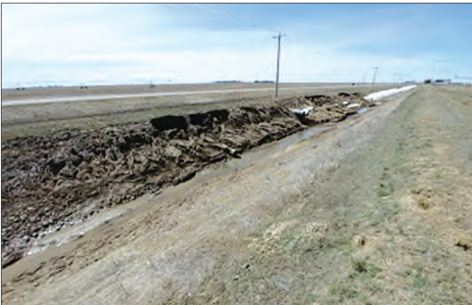
Figure 1.1: Major Slough on South Bank of Lateral G Big Bend Canal Due to Overland Flooding
