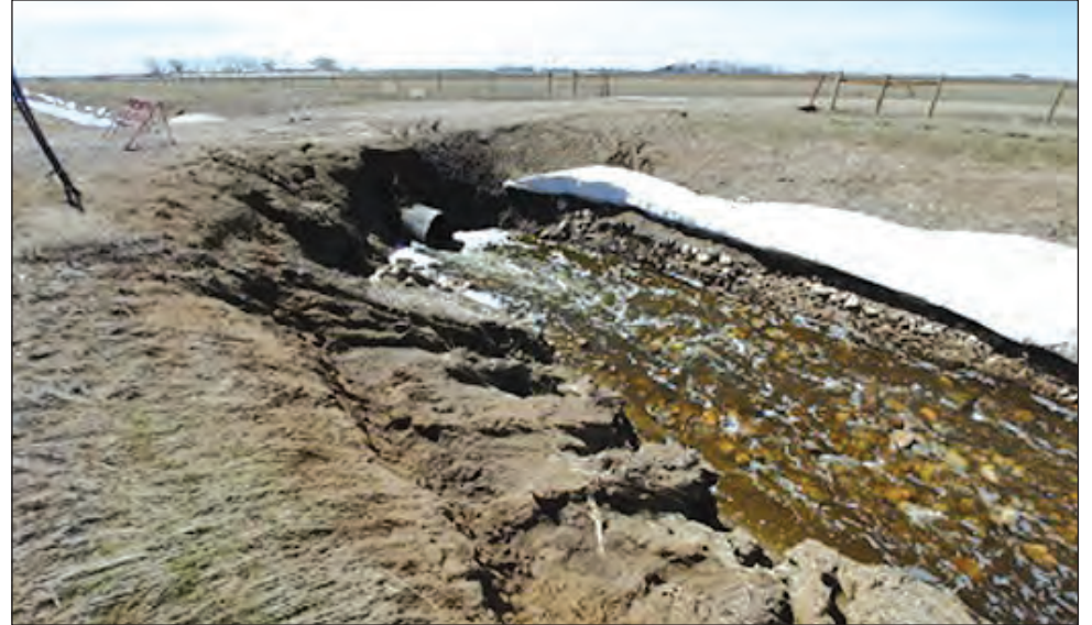
Figure 2.2: Piping Failure and Bank Sloughing at Lateral G-7 Big Bend Culvert Crossing (from North)
