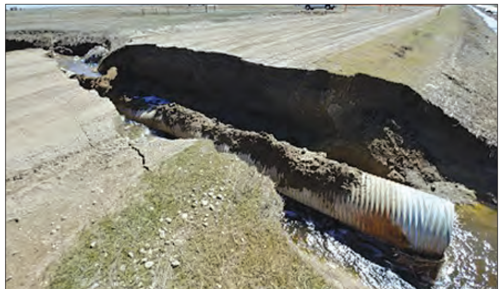
Figure 2.6: Lateral G-7 Big Bend/Range Road 16-1 Culvert Crossing Washout
