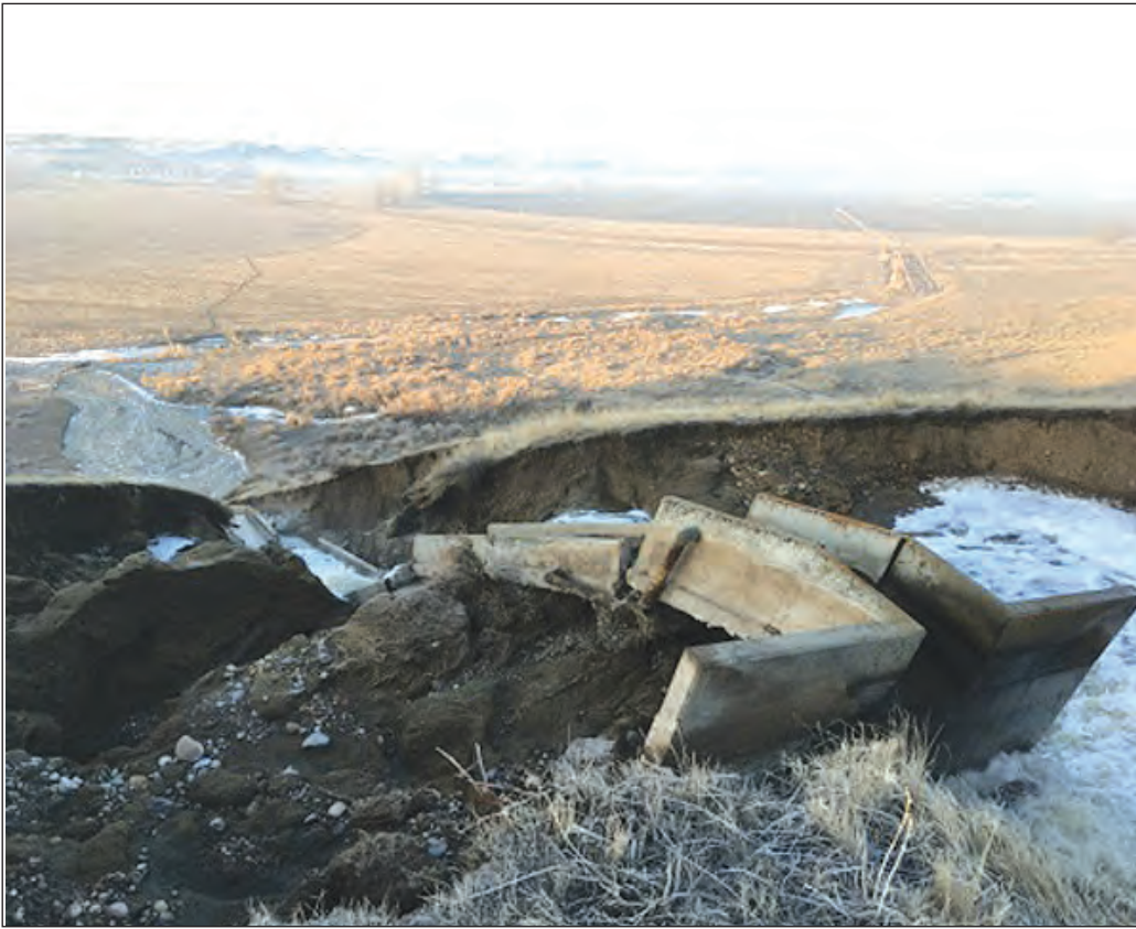
TOP: Damage to Bow River Irrigation District (BRID) infrastructure
