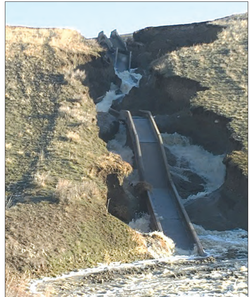
Damage to Bow River Irrigation District (BRID) infrastructure
