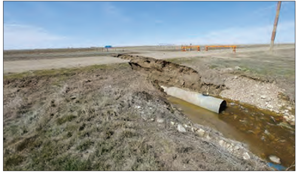
Figure 2.4: Lateral G-7 Big Bend/Range Road 16-1 Culvert Crossing Washout
