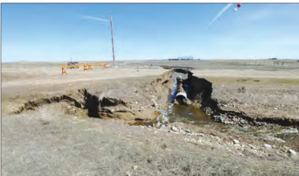
Figure 2.5: Lateral G-7 Big Bend/Range Road 16-1 Culvert Crossing Washout (from West)
