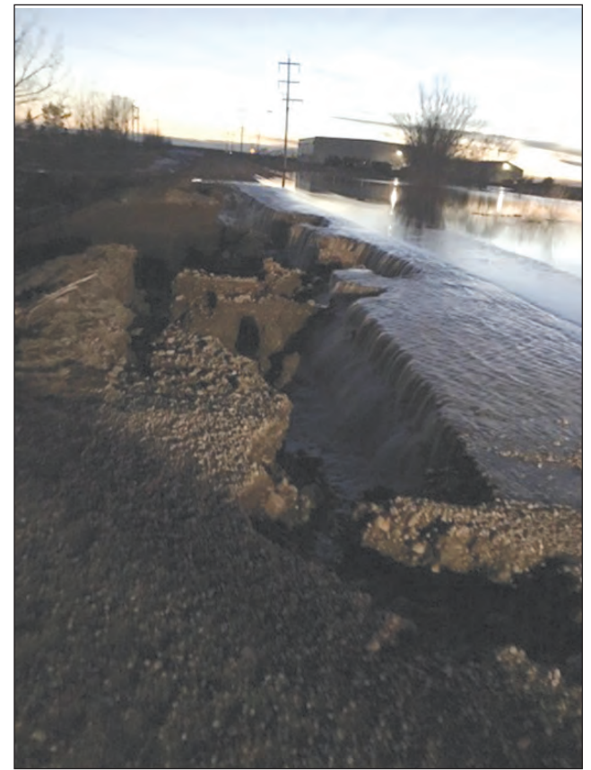
TWP RD 10-2 West of Taber Airport – Road washout
